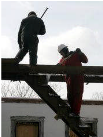
Figure 1 STAFF PHOTO BY JAN UNDERWOOD Workers prepare to take a staircase out of a house at 38 S. Horton St. in Dayton.
